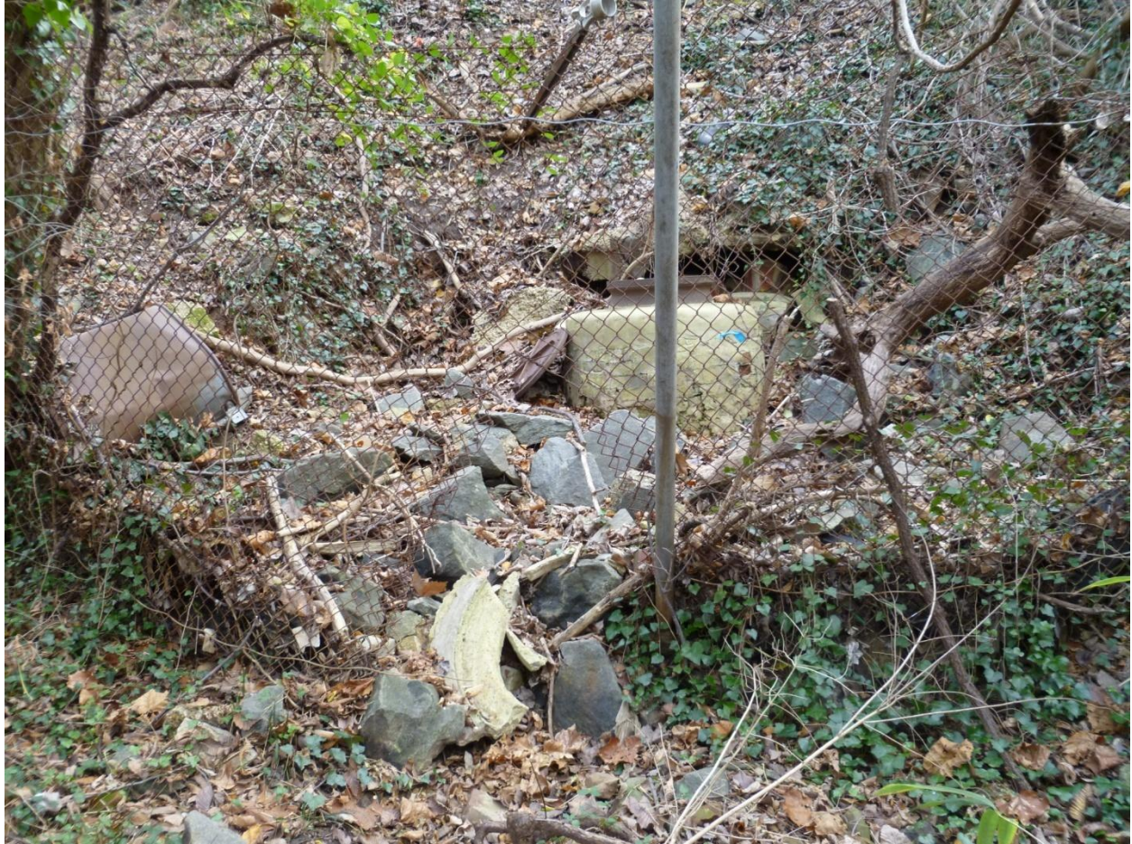
Sewer manhole located down slope of Jelleff. In spite of the solid waste debris used to minimize erosion, the soil upslope of the manhole has been eroded. If the round disc leaning against the manhole is the cover, this manhole may still be discharging into the park, i.e. this cover may not be bolted down to prevent discharge. (11-20-2011 photo)
