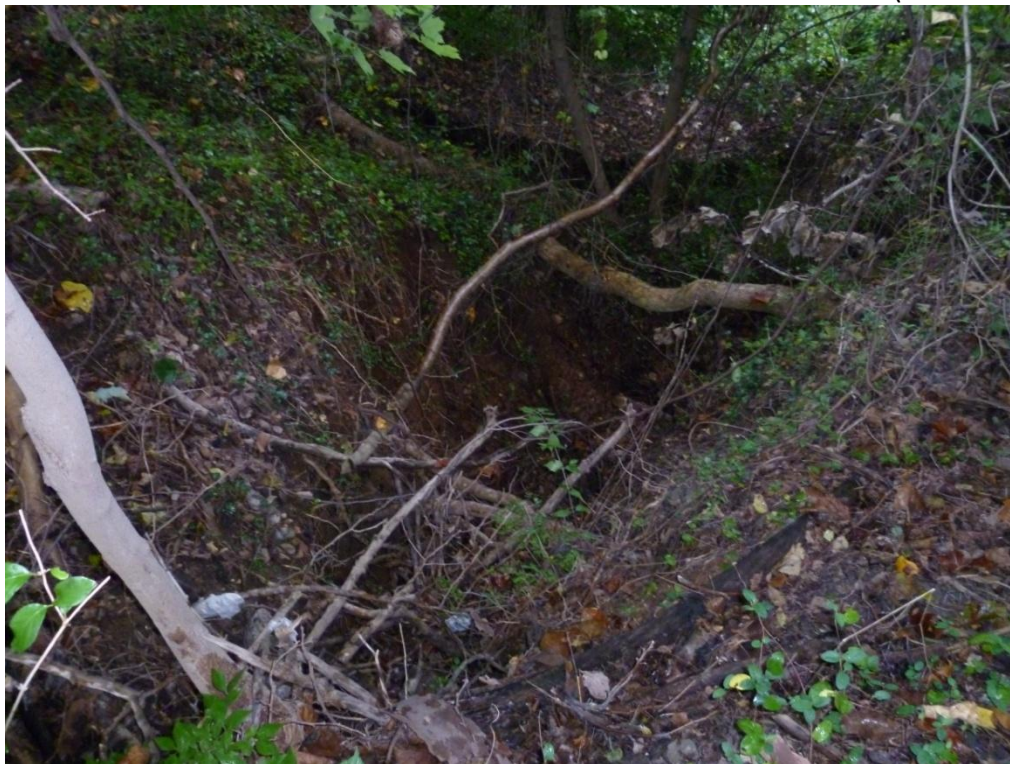
The above photo shows a gully from runoff leaving the Embassy of New Zealand property leaving the park fencing horizontal (visible at the top of the 10-1-2011 photo).
